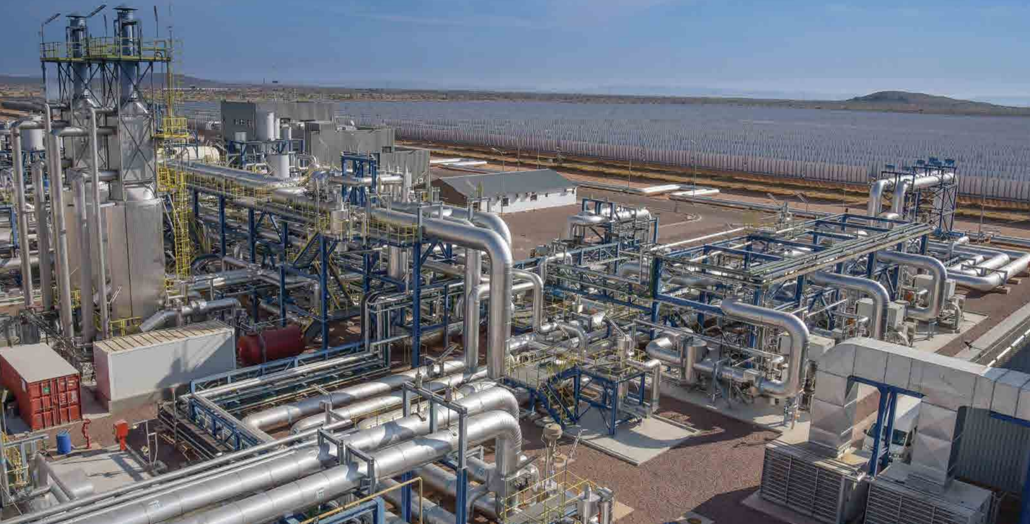
In the central plant the heat from the oil circulated around the mirrors is used to create high pressurised steam and to charge up the storage tanks of melted salt. The steam drives the 50MW turbine and the salt is stored to be used at night to carry on heating steam. Photo: Christy Strever
