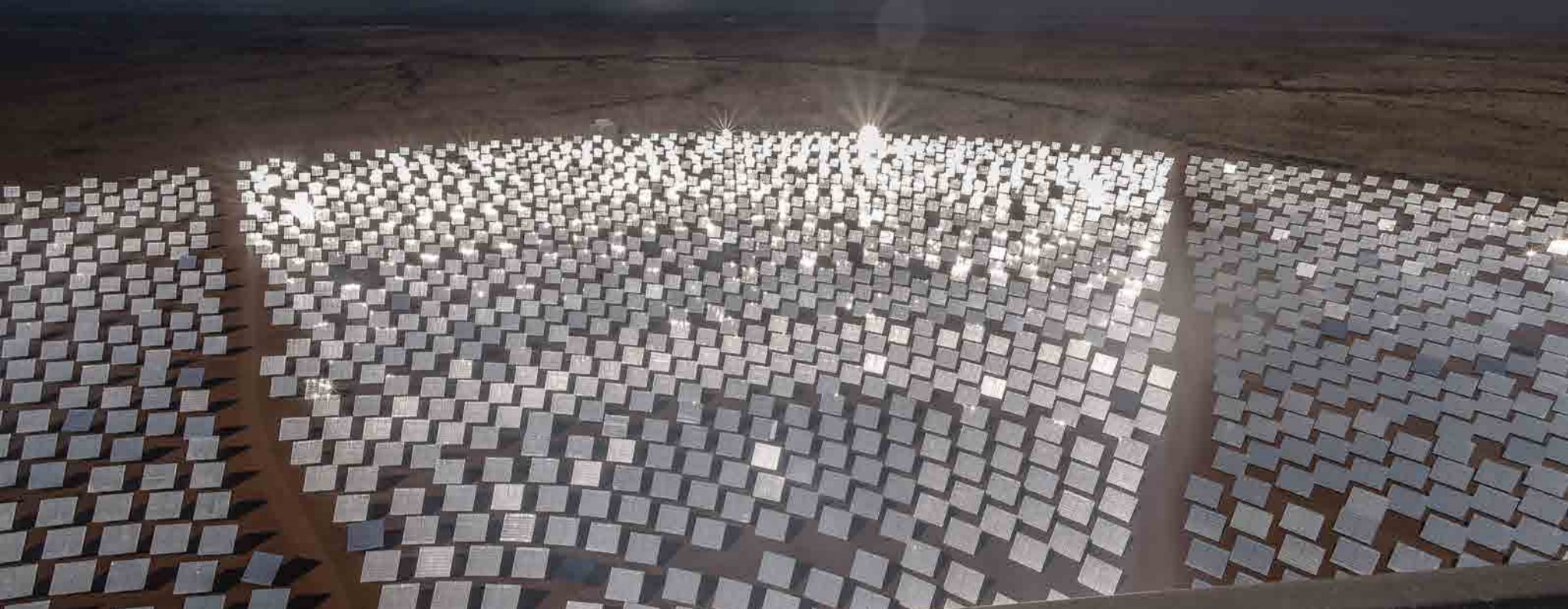
This picture was taken from the top of the tower and shows the array of mirrors below it. Photo: Christy Strever
