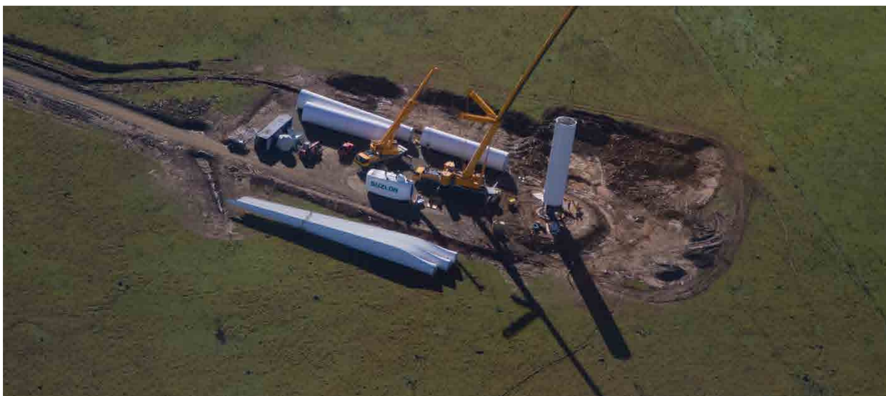
During construction, large cranes are used to assemble the tower and blades. Photo: Supplied by IPP Office
