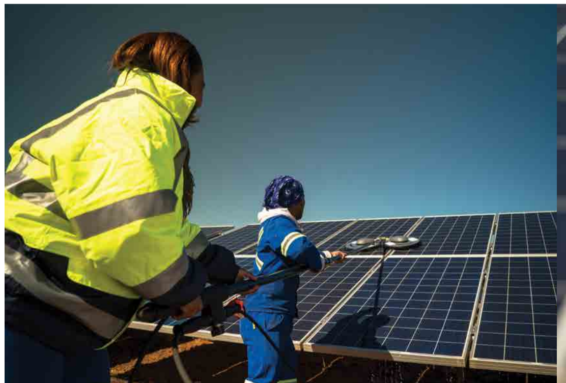
Workers conduct cleaning and maintenance work at the 96MW Jesper Solar Photovoltaic Power Plant in the Northern Cape.
