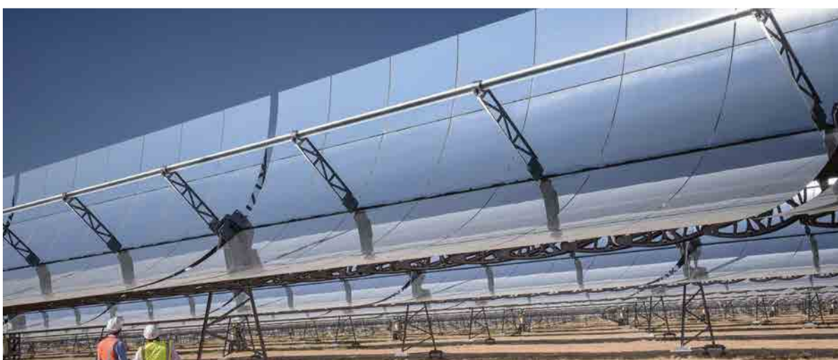
In the central heat collector element is a high temperature oil that absorbs the sun's heat, reaching 393°C as it circulates around the mirrors. Photo: Christy Strever
